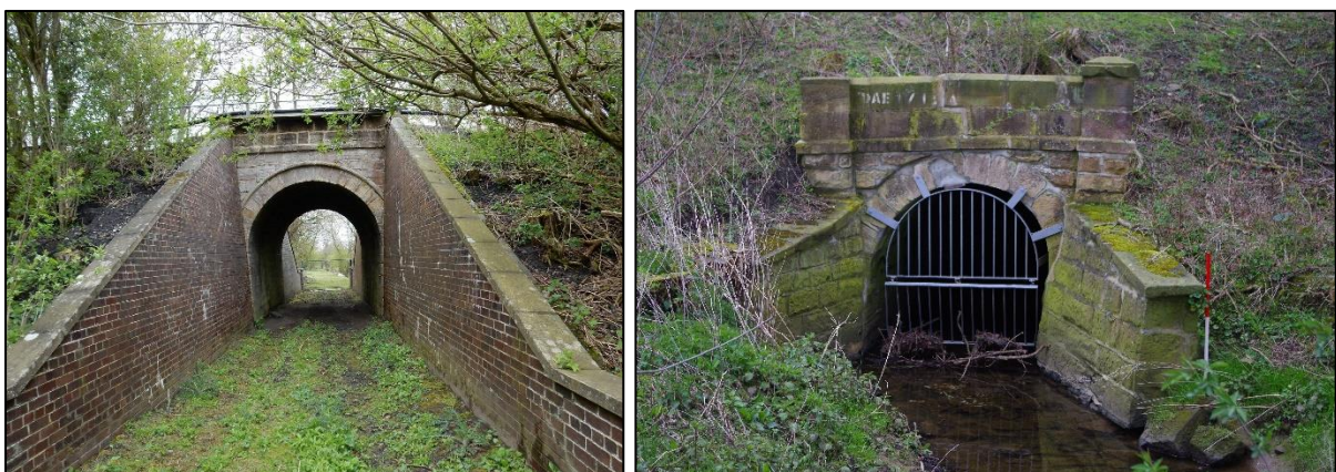
Plate 3. Accommodation bridge with renewed wing walls (left) and culvert adjacent carrying Dene Beck (right).
