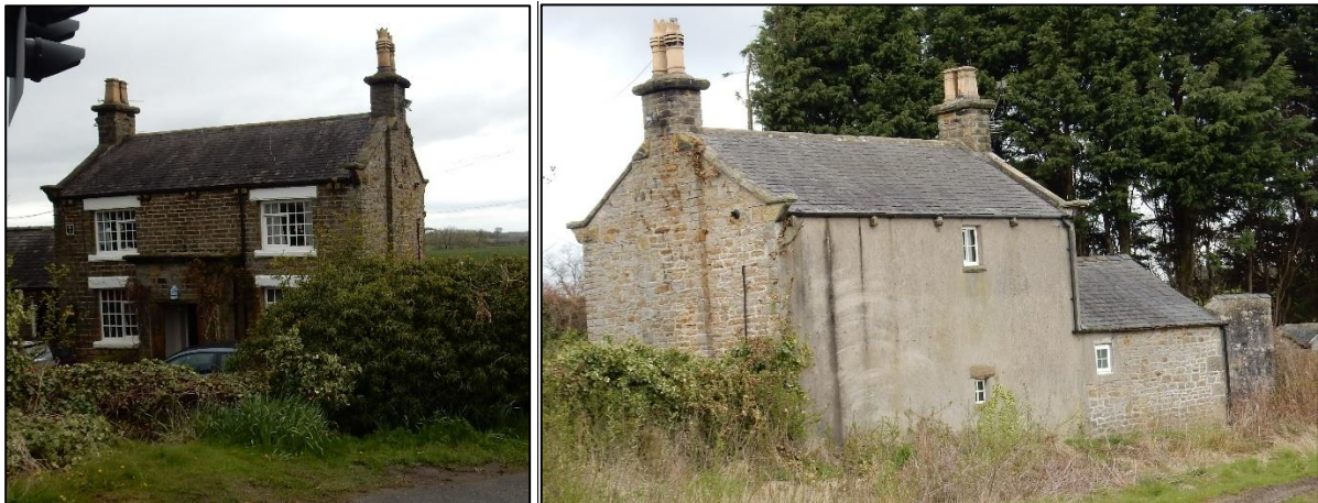
Plate 2. The Crossing Keeper's Cottage at Whiley Hill front elevation facing the line (left) and rear elevation facing fields (right)
